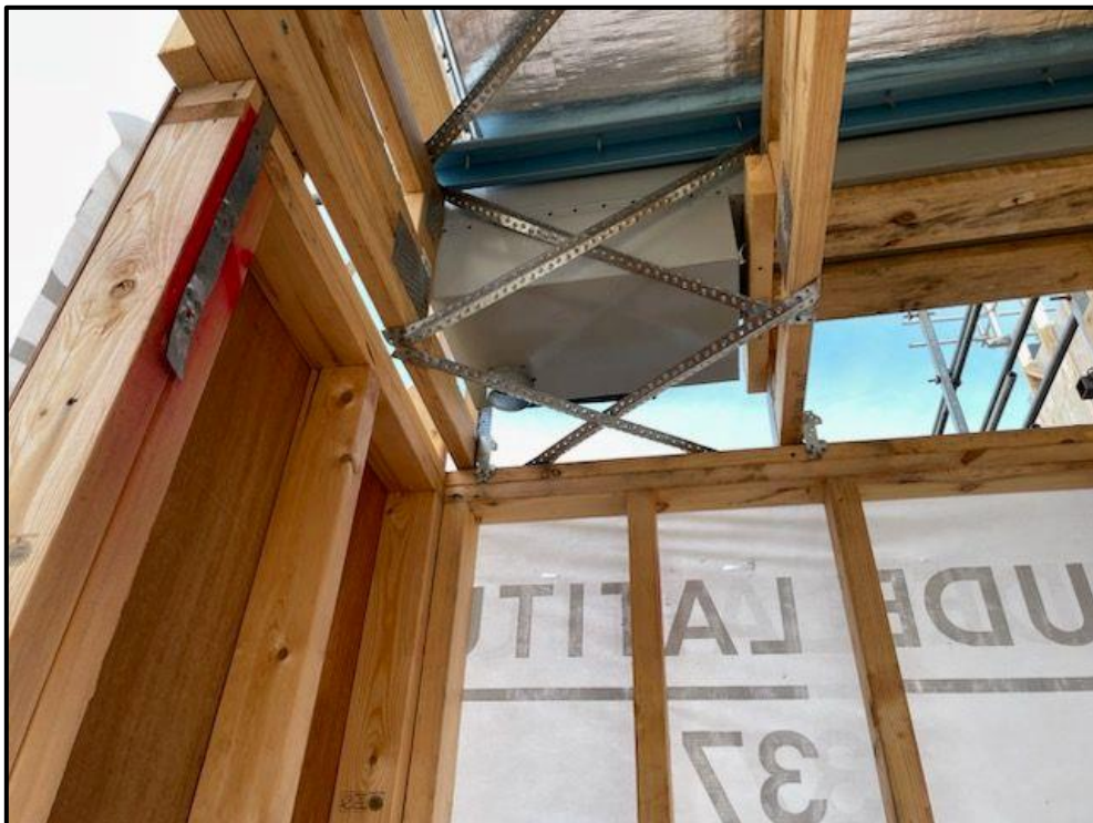
Photograph 6 – Type A overflow
