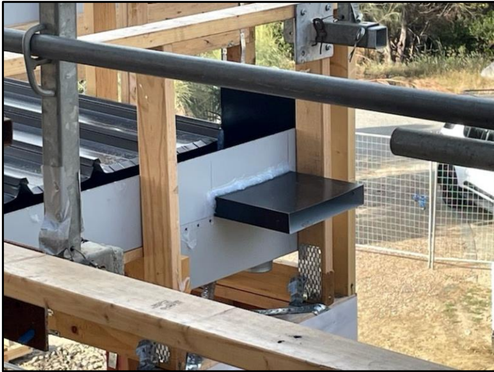
Photograph 4 – Type A overflow
