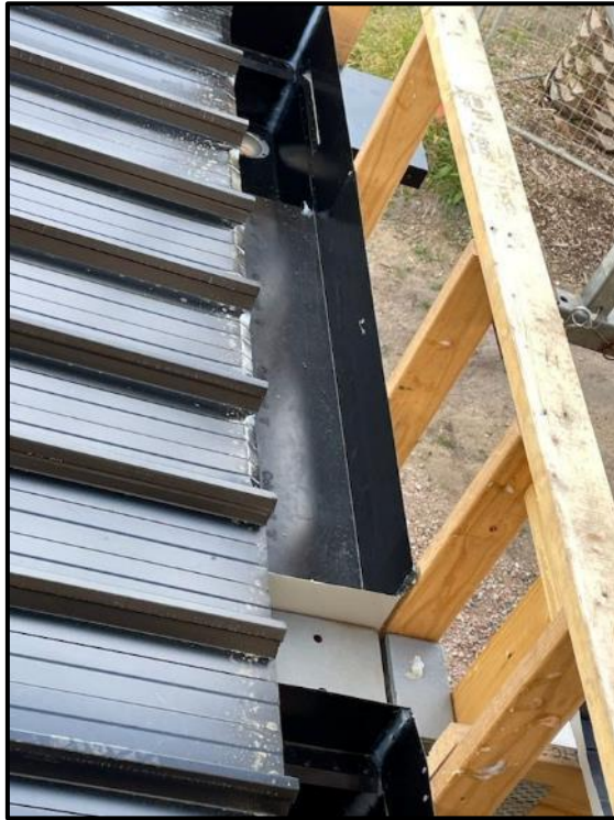
Photograph 5 – Type A overflow
