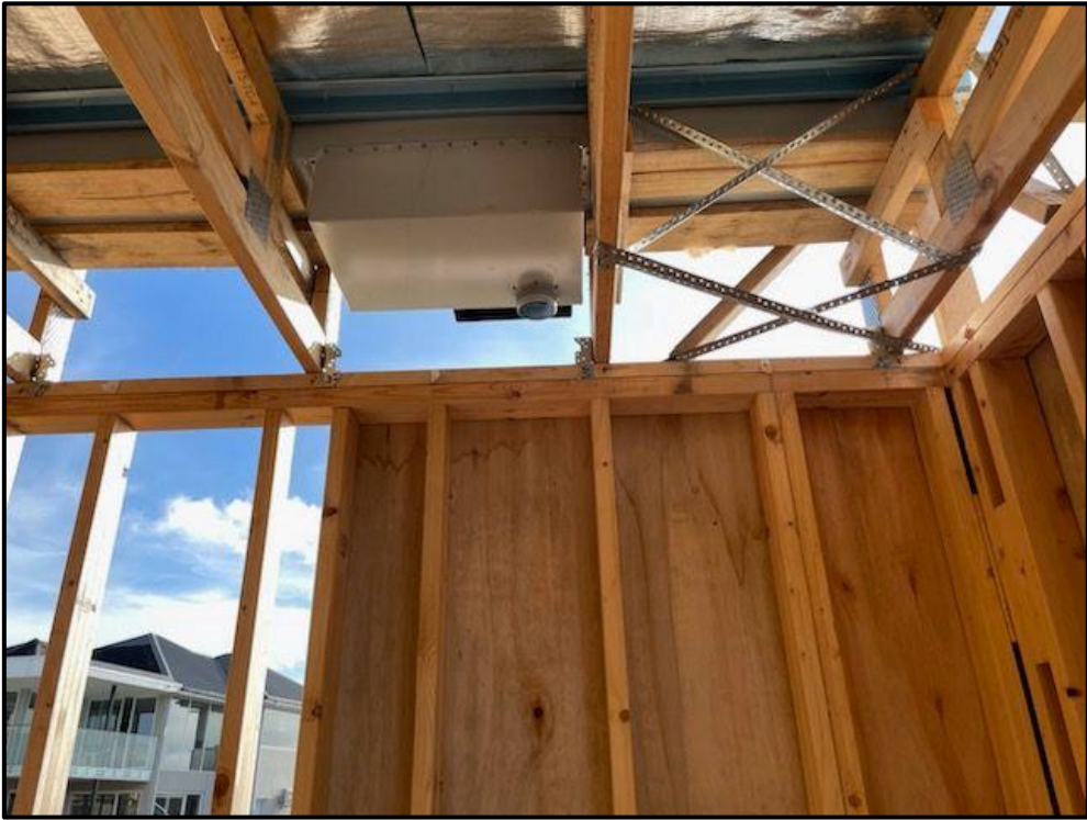
Photograph 3 – Type A overflow
