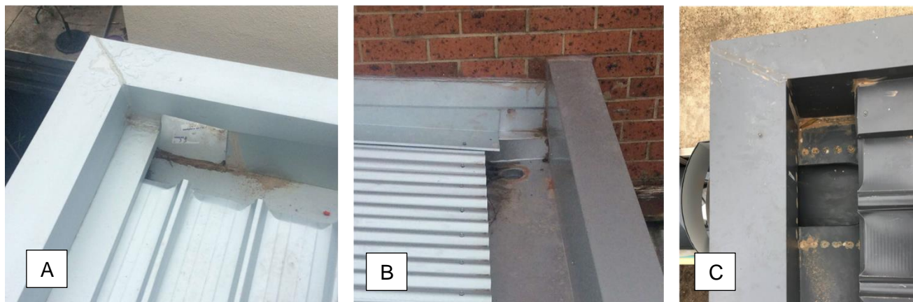
Image 1: Examples of non-DtS box gutter installations
