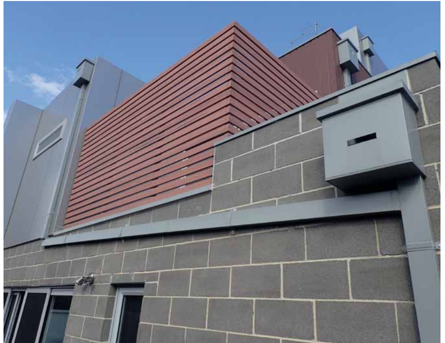
Many housing estates have upwards of five rainheads - most of which are not compliant
